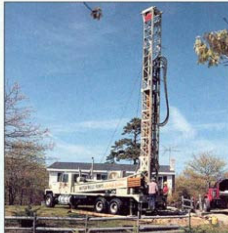
TH-60 Cyclone drill has 32,500-lb. (14,742-kg) pullback; retractable hydraulic tophead; pipe carousel inside derrick; exclusive I-R power transfer; air, mud or foam systems.
